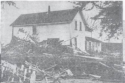
FIVE PEOPLE PASSED THE FLOOD CREST IN THIS ISLAND DISTRICT RANCH HOME TUESDAY NIGHT, DECEMBER 22. They were Mr. and Mrs. Ray Tedsen and three children, who took refuge in the second floor, where the flood waters also reached. The entire first floor was wrecked and for awhile they feared the house was about to float away. Part of the Bahnsen home, which was swept from a mile distant, lodged against the side of this home. The Ray Tedsens are salvaging what they can and will burn what is left, moving to the large home, soon to be vacated by the senior Fred Tedsens, who are moving to Ferndale. The latter also had a hectic night and were not rescued until 2 p.m. Wednesday.
